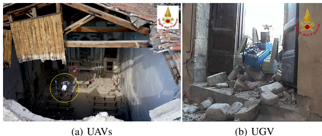
Fig. 1. UAVs and UGV of the TRADR project after the earthquake in Amatrice / Italy 2016.
